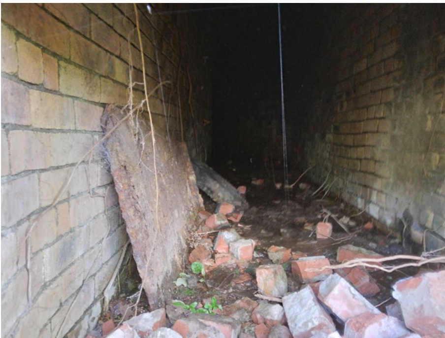
Plate 31: Tunnel under the site of the Plas-Kynaston Foundry, looking east (outside the Site)
