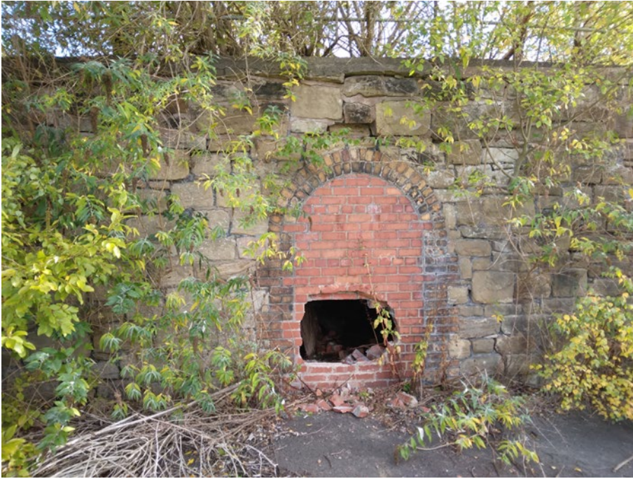
Plate 30: Close-up of late 19th-century retaining wall of Plas-Kynaston Foundry, c. 10m to the east of the Site, looking east
