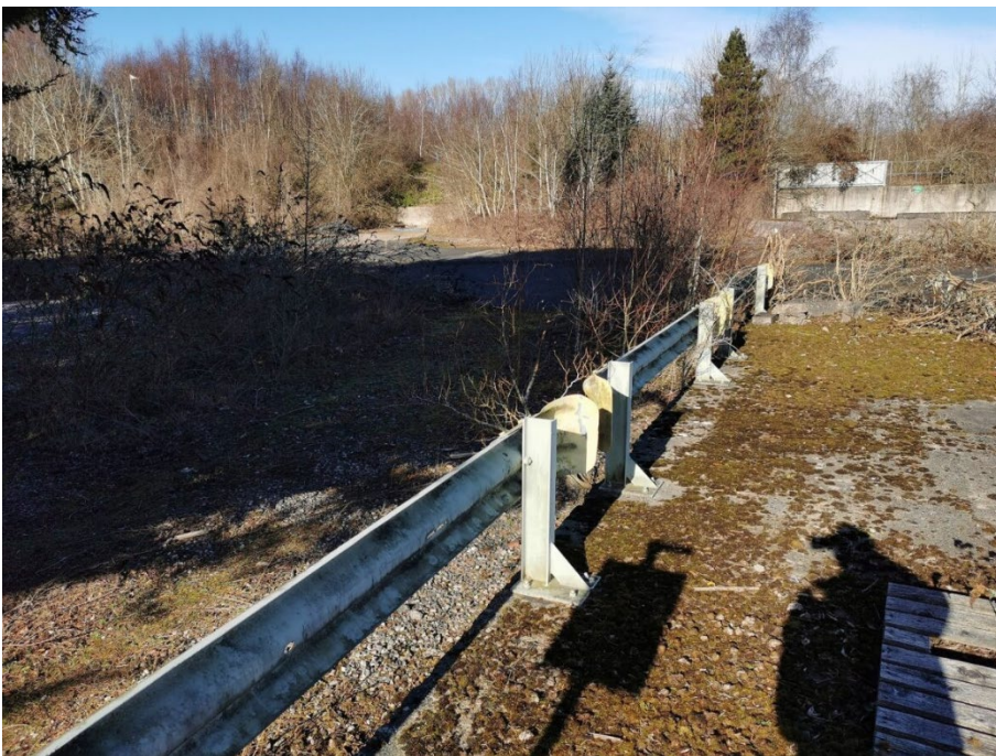
Plate 7: Surviving 20th-century railings and walls in southern part of Site, looking north
